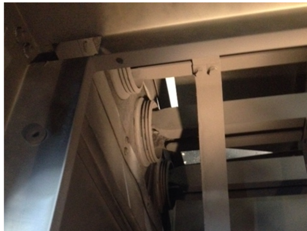
Figure 1. Scorched 21 kV busbar.
